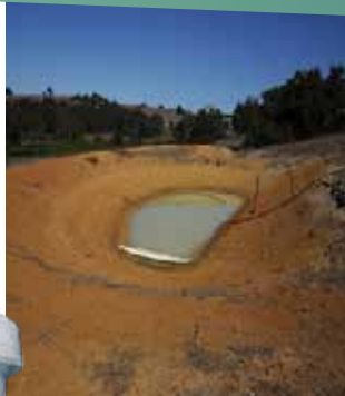
Leaking dam walls
